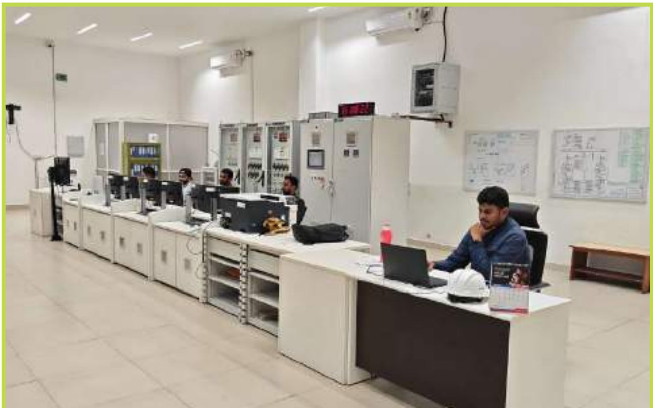
Power House Control Room
