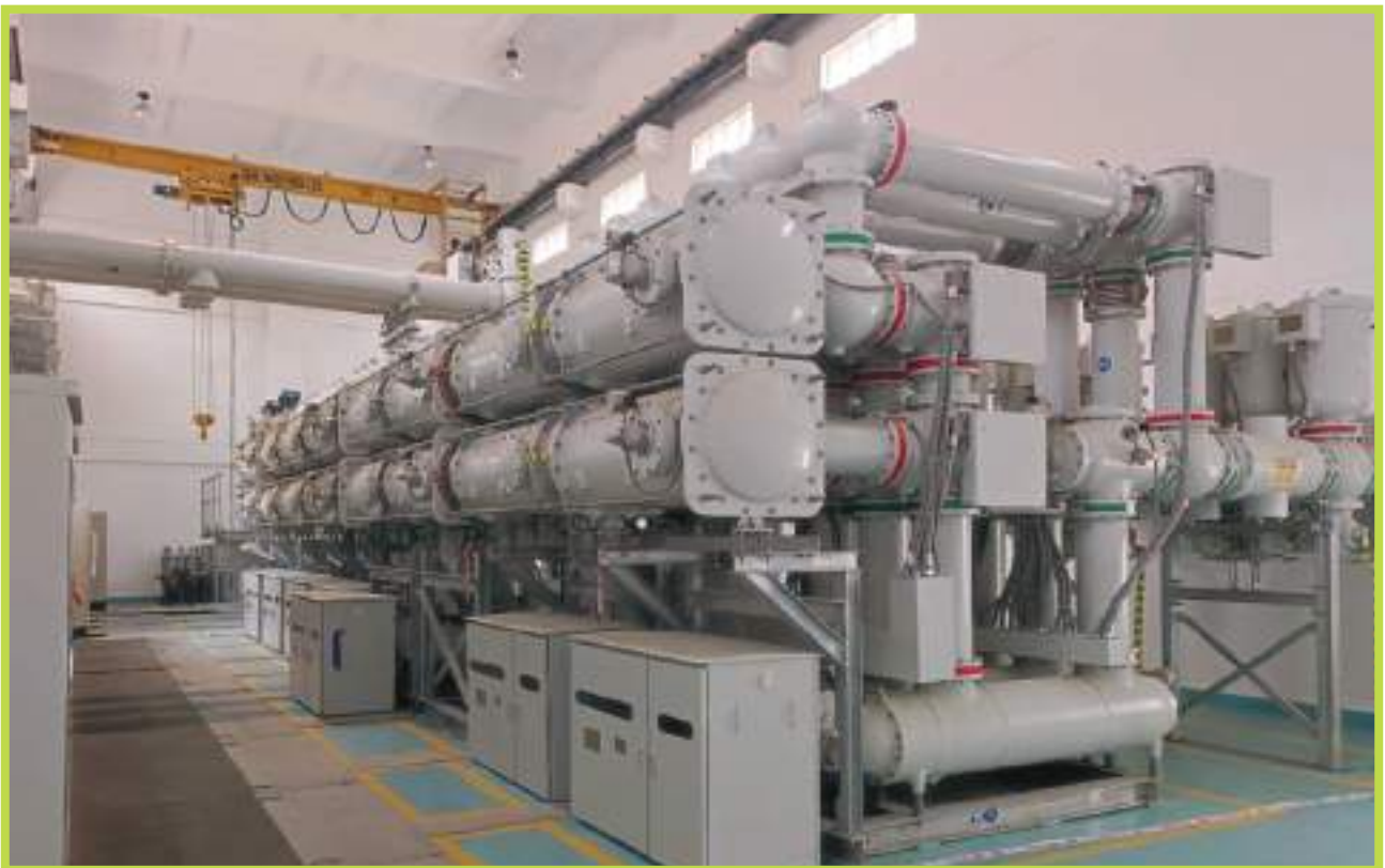
GIS Equipment at New Khimti Substation
